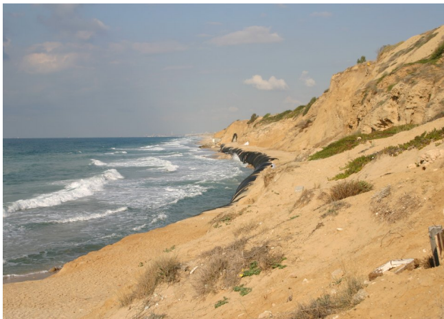
Figure 5. Coastal erosion protection using geotextile tubes filled with sand at northern Ashkelon coast.
