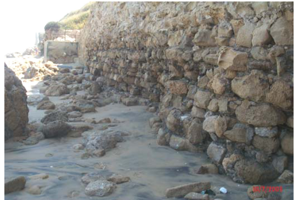
Figure 4. Detail of the damaged ancient wall at Ashkelon park.
