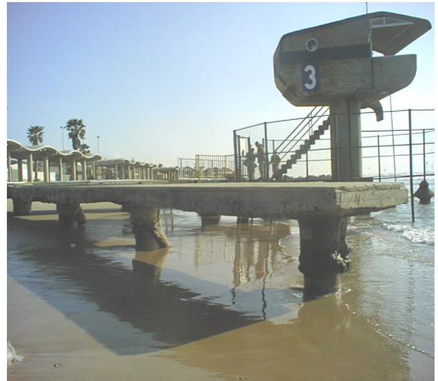
Figure 12. Severe depletion of beach sand at Haifa Dado beach, (see missing sand below walkway).
