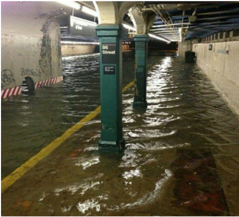
Figure 8.4. Hurricane Sandy causes flooding in New York City's subway (86th Street Lexington Ave. Station, Upper East Side in Manhattan). Source: https://www.pinterest.com/pin/218143175672242767/ .
